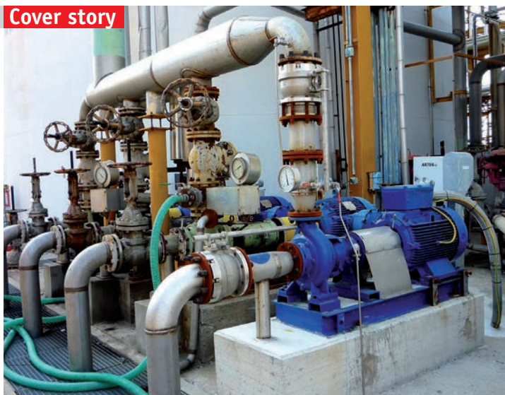
RD pump (ISO 5199) installed in a urea plant
